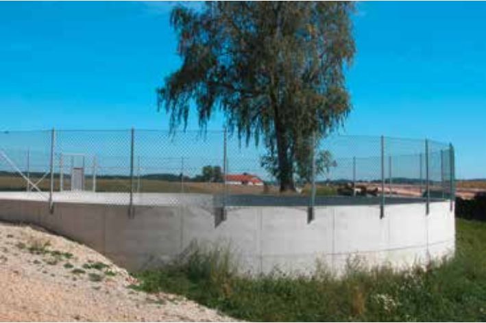
Circular storage tanks for slurry and wastewater management in modern livestock operations
