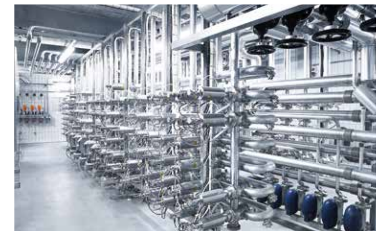
CIP system for automated cleaning and maximum hygiene
